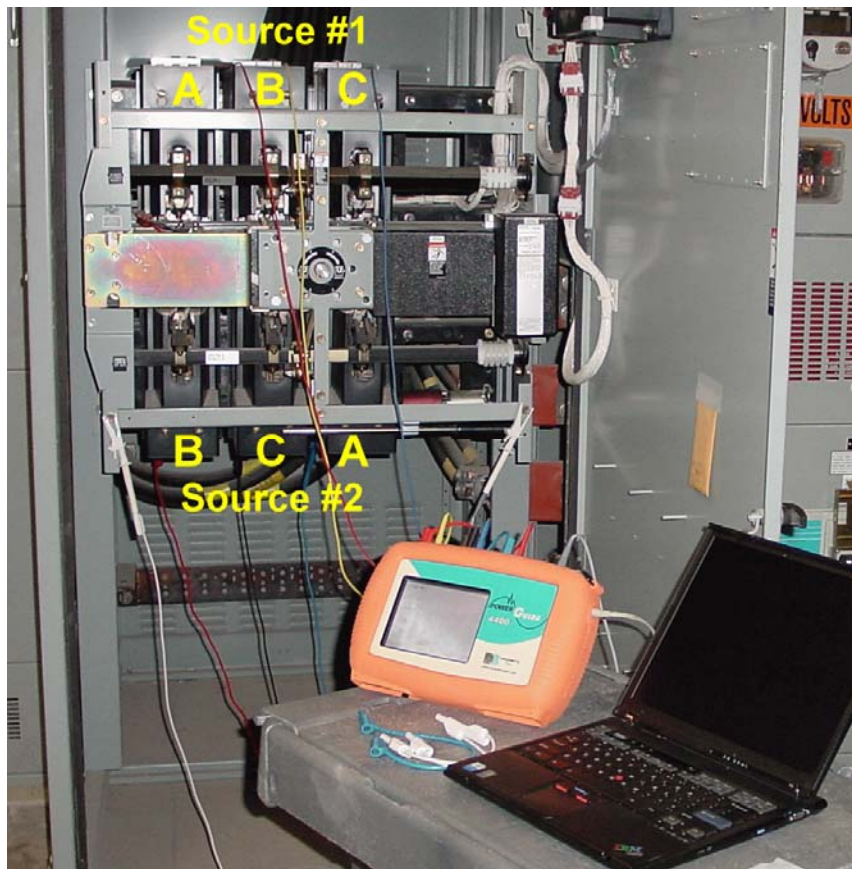
Photo 2 - New transfer switch showing phase termination rotation between sources.
