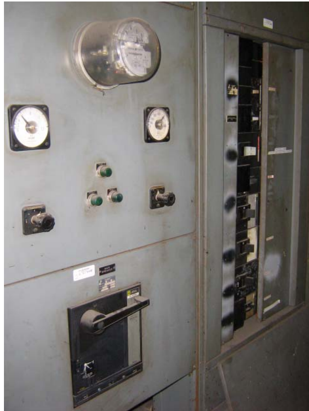
Photo 2 – SWBD NO. 3 is a 480V 3P3W 1200Amp supply.
