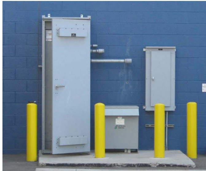
Photo 1 – Panelboard DB1 3P4W 480/277Vac 800A.
