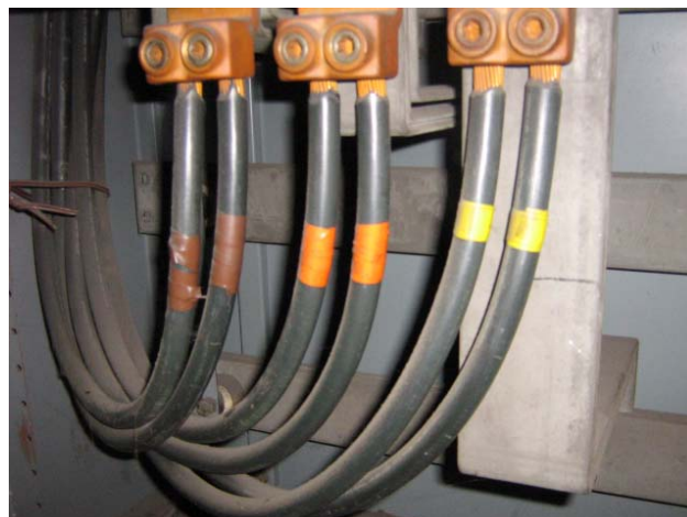
Photo 3 – SWBD 3 showing tap off main breaker.
