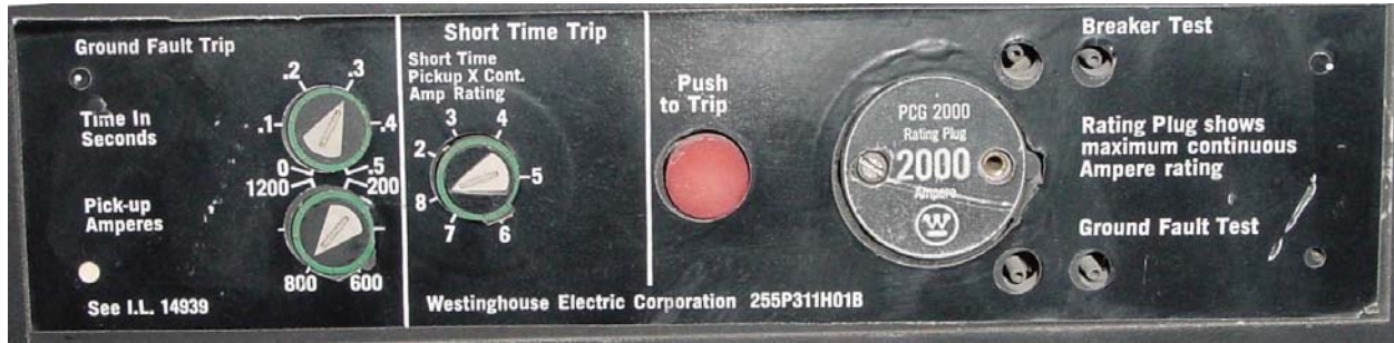
Photo 3 - Main 2000A breaker ground fault and short time trip settings.
