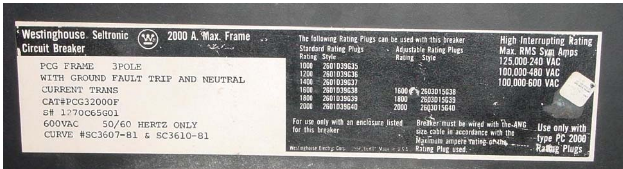
Photo 2 - Main 2000A breaker name plate.
