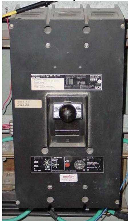
Photo 1- Main 2000A curcuit breaker.
